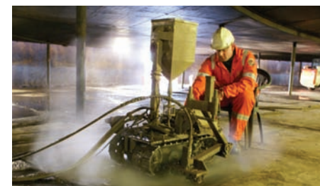
Safe-Cut uses a Jet Edge-powered robotic water jet system to remove old floors from storage tanks.
